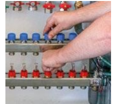
8. Open all valves and flow meters. Install the sealing caps and open the ball valves.
