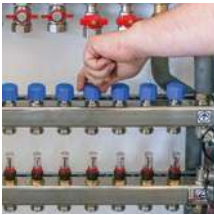
5. Open the valve for the circuit to be flushed and close all other valves. Turn on the water supply.
